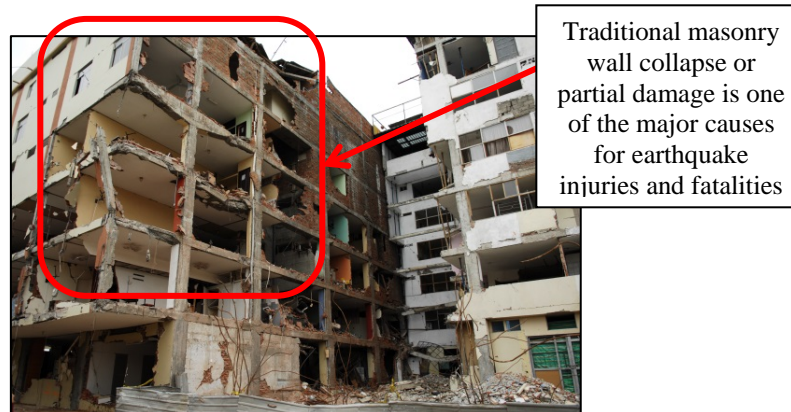
Fig. 1. Overbalanced brick masonry recorded during the 2016 Ecuador earthquake occurred on April 16, with a moment magnitude of 7.8 and a maximum VIII severe Mercalli intensity. Adapted from [6]
