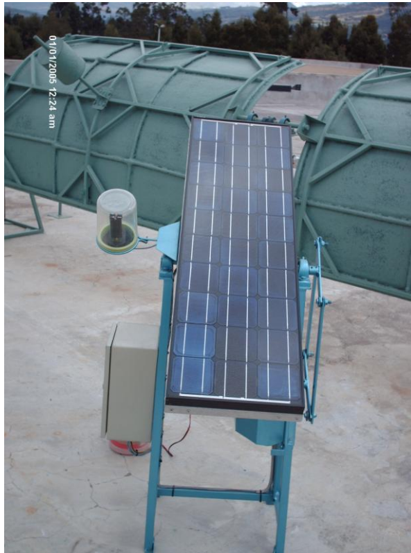
Figura 2.14. Panel fotovoltaico de 43 Wp
