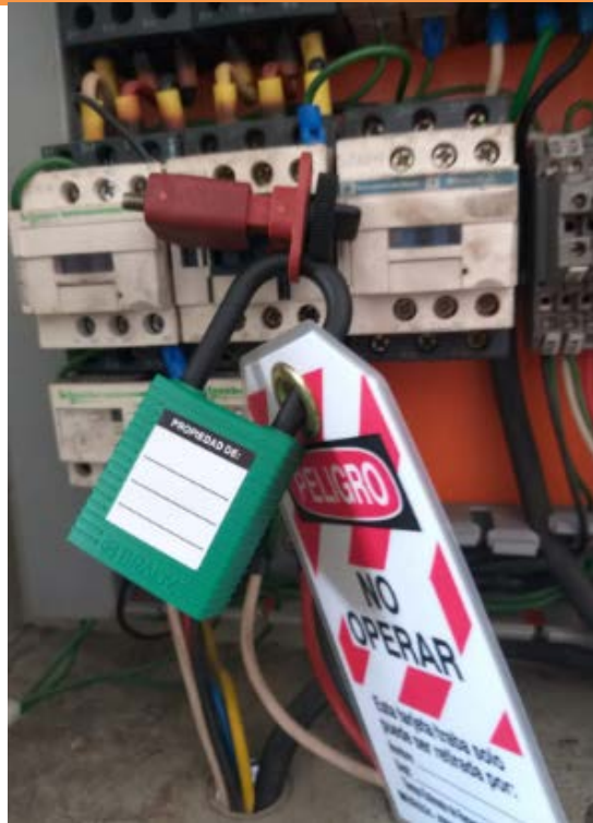
panel principal de control de bombas 3HP
