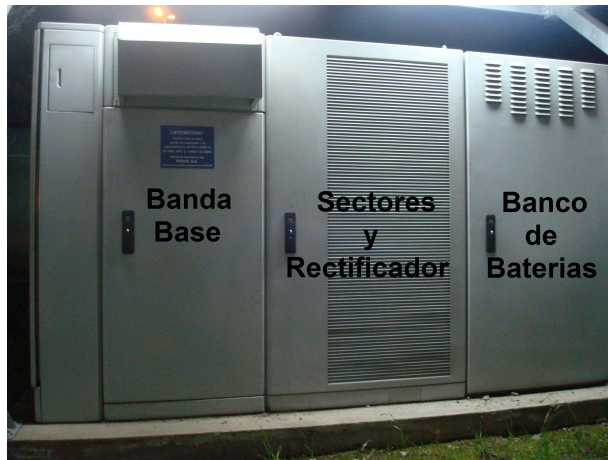
Figura 2.20: BTS CDMA Nortel Networks
