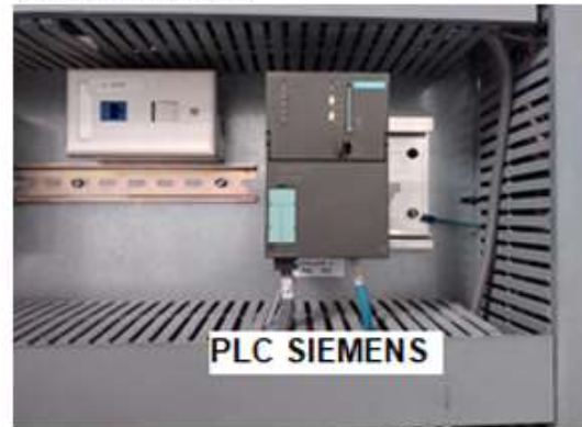
Maestro PLC Siemens.
