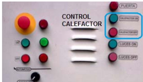
Figura 3.37: Control de calefactor
