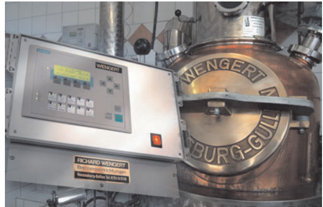
Transparent distillation process thanks to clear display on SIMATIC C7
