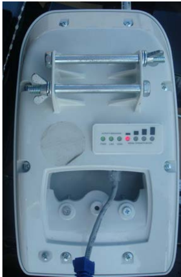
Figura 4.56 Power Station 2EXT, cerro Cabuyas,
