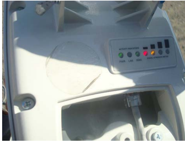
Figura 4.54 Power Station 2EXT, Cerro Animas.
