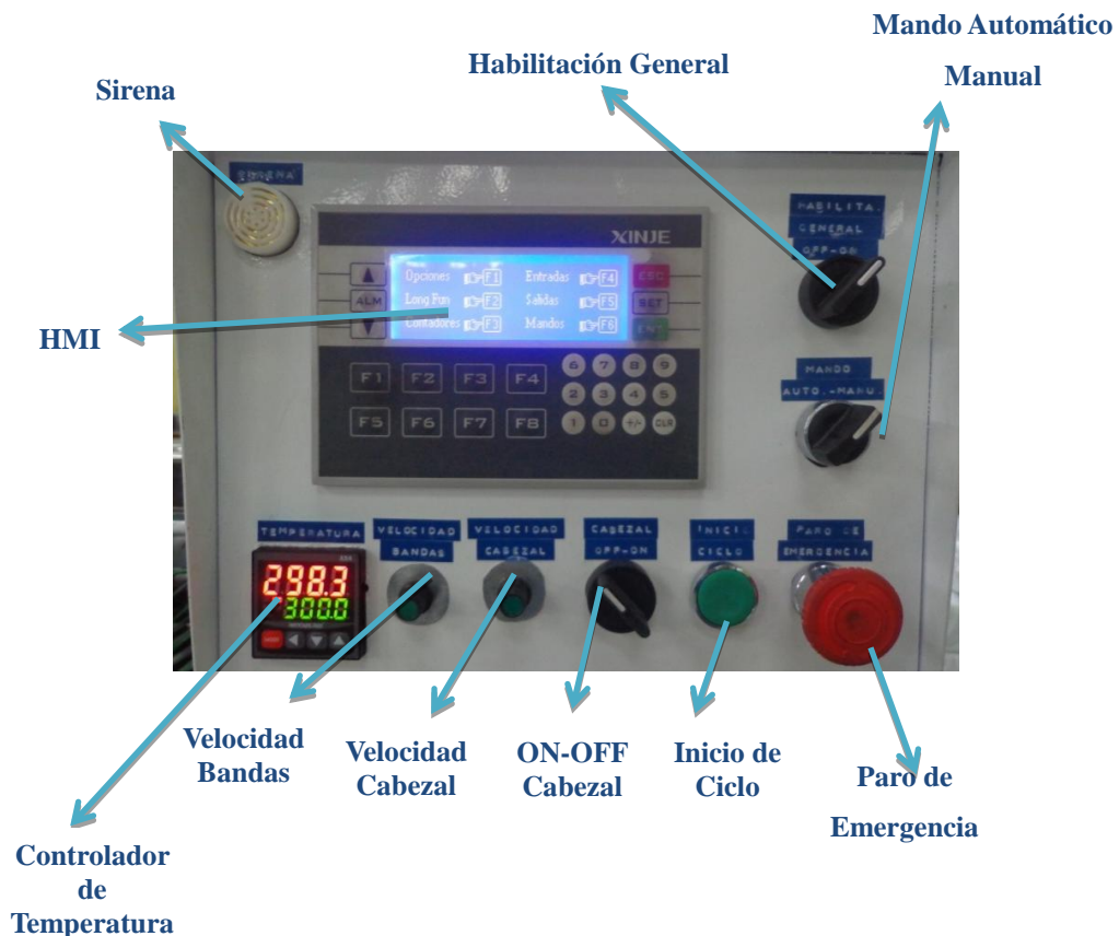
Figura2. 38: Tablero de Control
