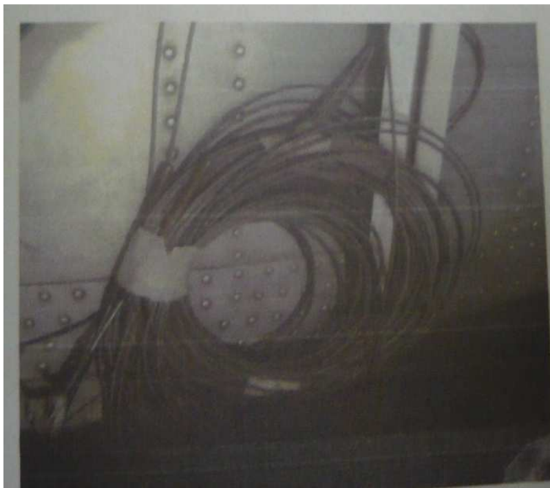
Figura 3.14: Cables de control enrollados
