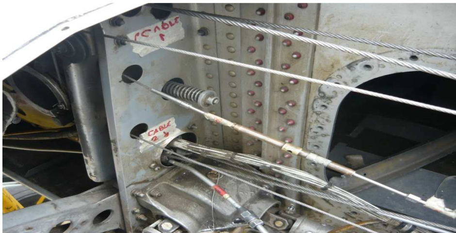
Figura 2.27: Cables de control
