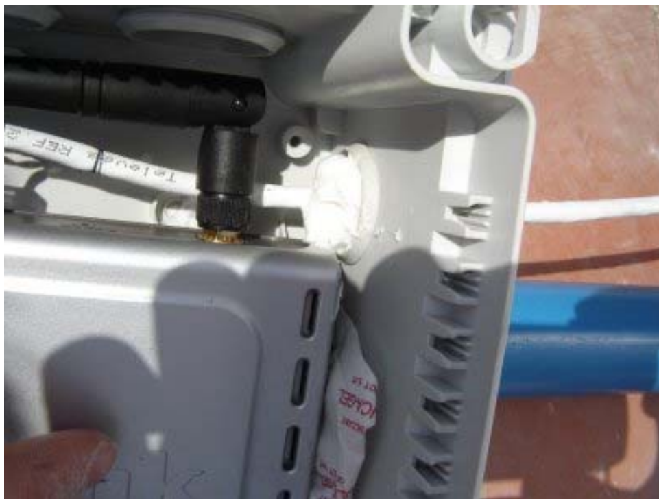
Figura 4.52. Access Point instalado
