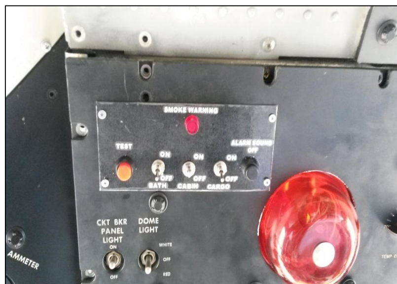
Figura 42: panel de smoke warning
