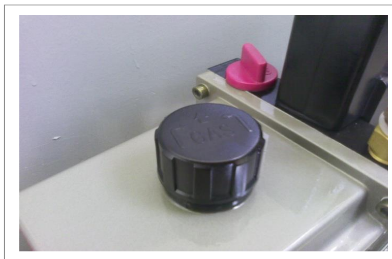
Figura 3.11 Escape de gas
