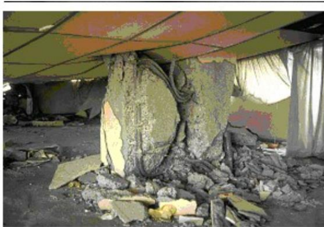
Falla del Hotel Terminal Guatemala, 1976
