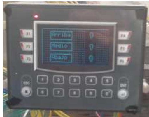
Figura 5.3. PLC Renu Electronics
