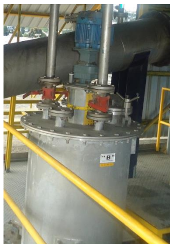
Figura 7 Tanque TQ_01, Reactor MQ6
