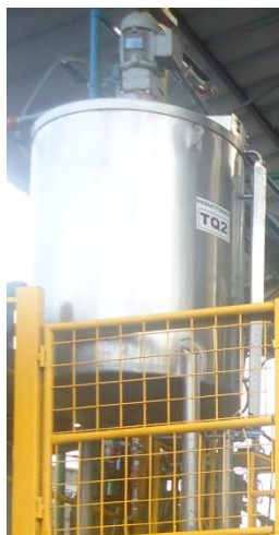
Figura 6 Tanque TQ_02, Reactor MQ6
