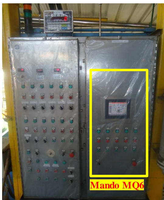
Figura 23 Tablero de control Reactor MQ6, mando MQ6
