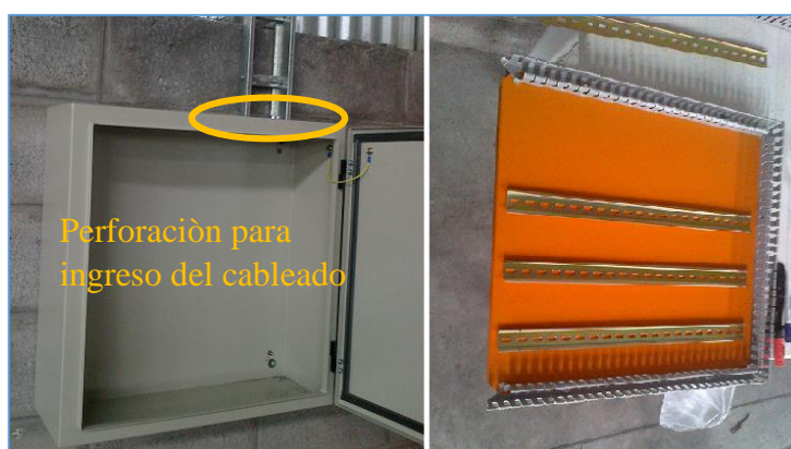
Figura 4-4 Gabinete de control
