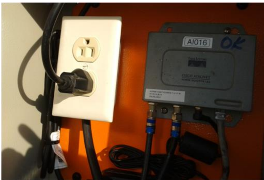
Figura 3.21 Power Injector de radio Cisco 1300
