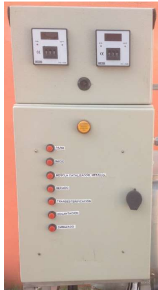
Figura 89 Panel de control del micro reactor.
