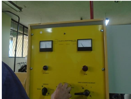
Figura No. 56. Tablero de control
