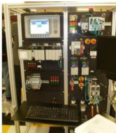
Figura 15. Sistema de entrenamiento Allen Bradley de "Electrical Engineering - University of Michigan"
