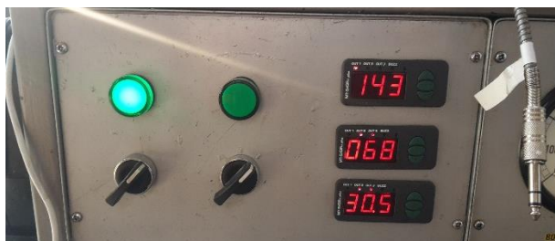
Figura 89 Panel de control del BPMV
