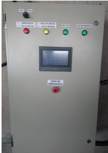
(a) Tablero de control vista exterior
