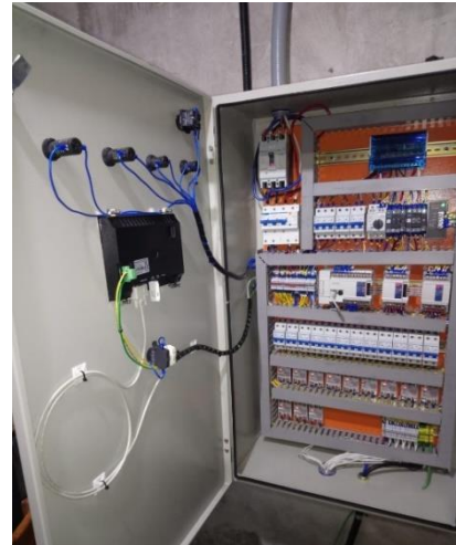
(b) Tablero de control vista interior
