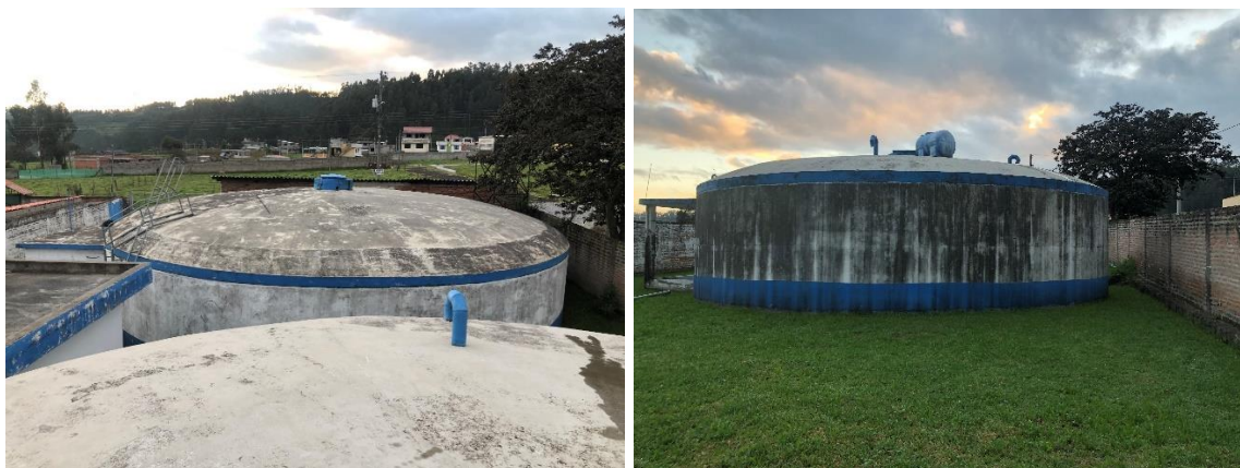
Tanques Carlos Gavilanes
