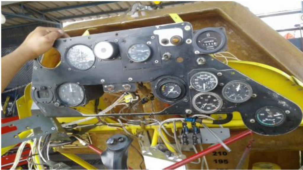
Figura 24: Main panel obsoleto
