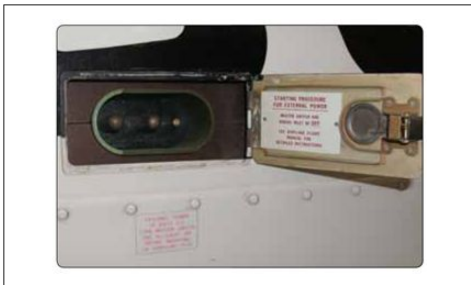
Figura 18. External power receptacle
