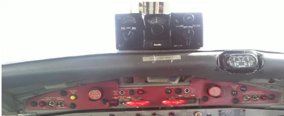
Figura 2.15: Panel de Fire protection.
