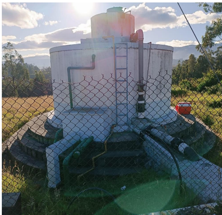
Tanque circular Cashapamba
