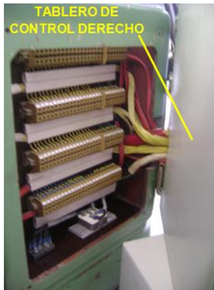
Figura 4.24: Tablero de control
