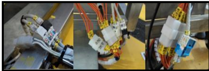
Figura 20: Borneras y jacks.
