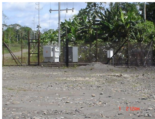
Foto No.9. Bombeo Electrosumergible
