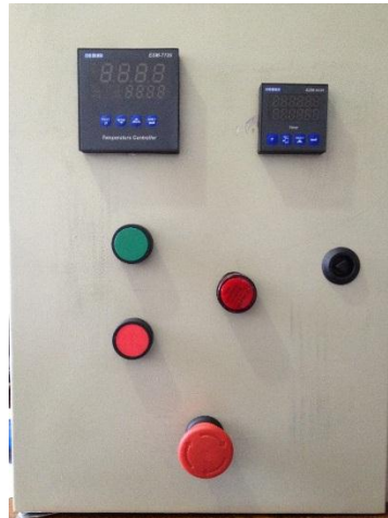
Figura 3. 11: Tablero de control. (Aguirre/Sánchez, Tablero de control 2013)
