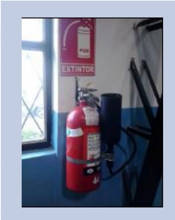
EXTINTOR A, B, C.
