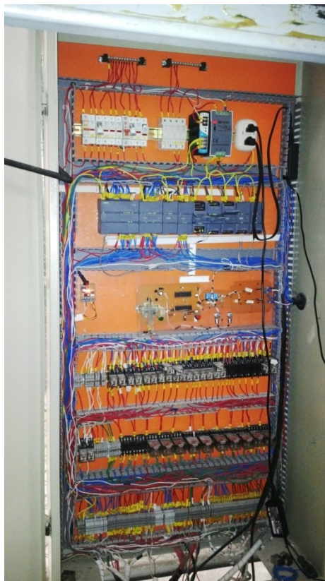
Figura 3.14 Tablero de control
