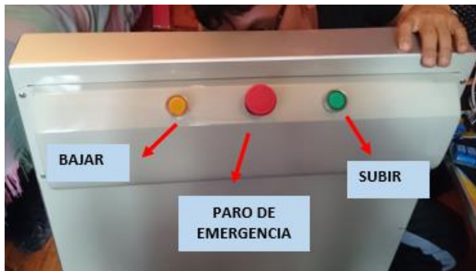
Figura 117. Panel de control principal.
