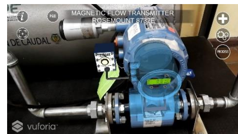
Figure 13. Calibration of the Rosemount 8732E transmitter
