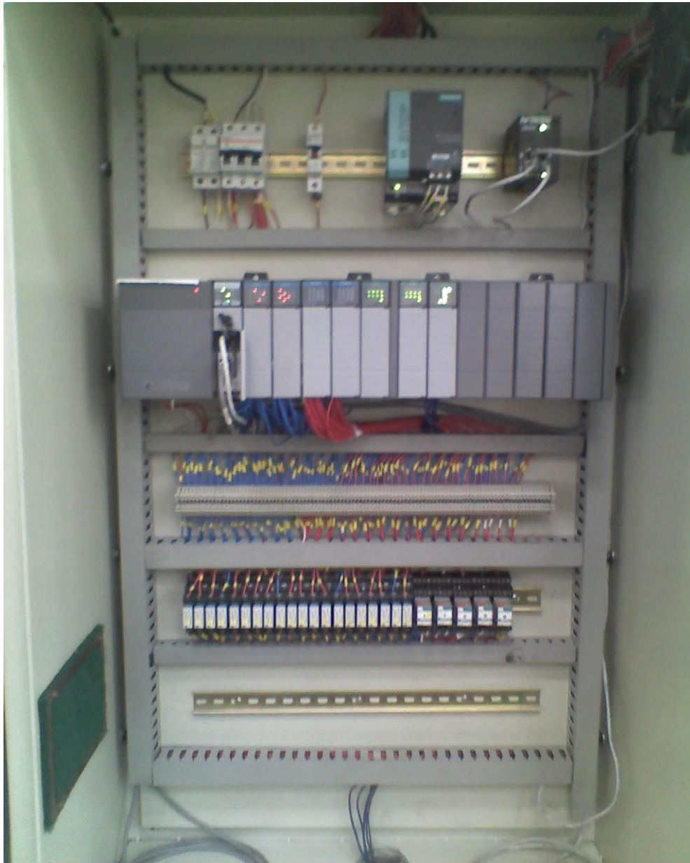
Fig. 3.16 Panel de Control Principal (vista interior).
