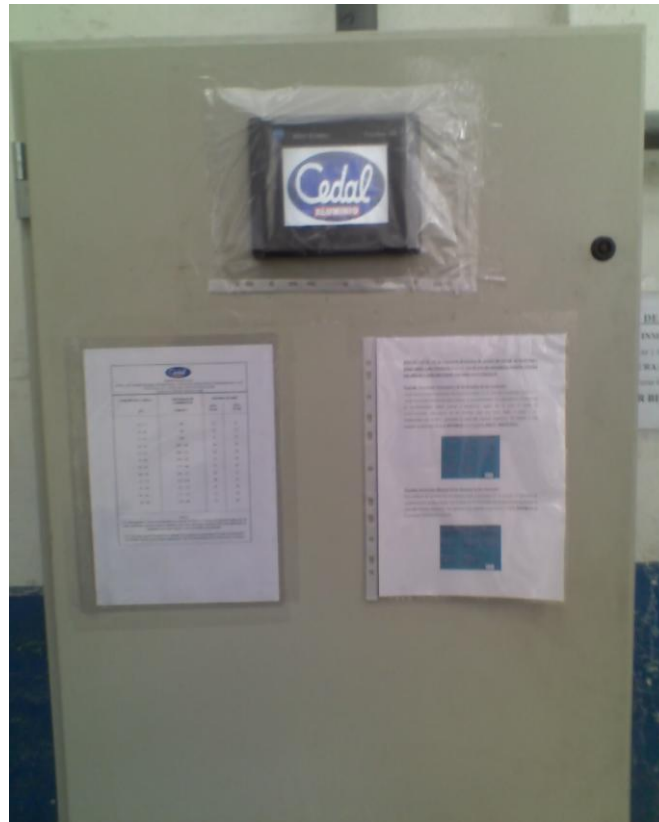
Fig. 3.15 Panel de Control Principal (vista exterior) y touch screen (parte superior).
