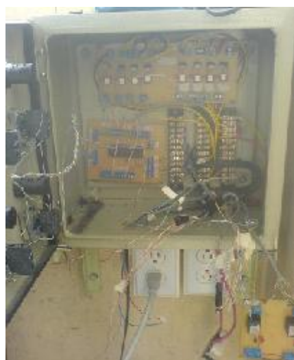
Figura 3.11 Tablero de control
