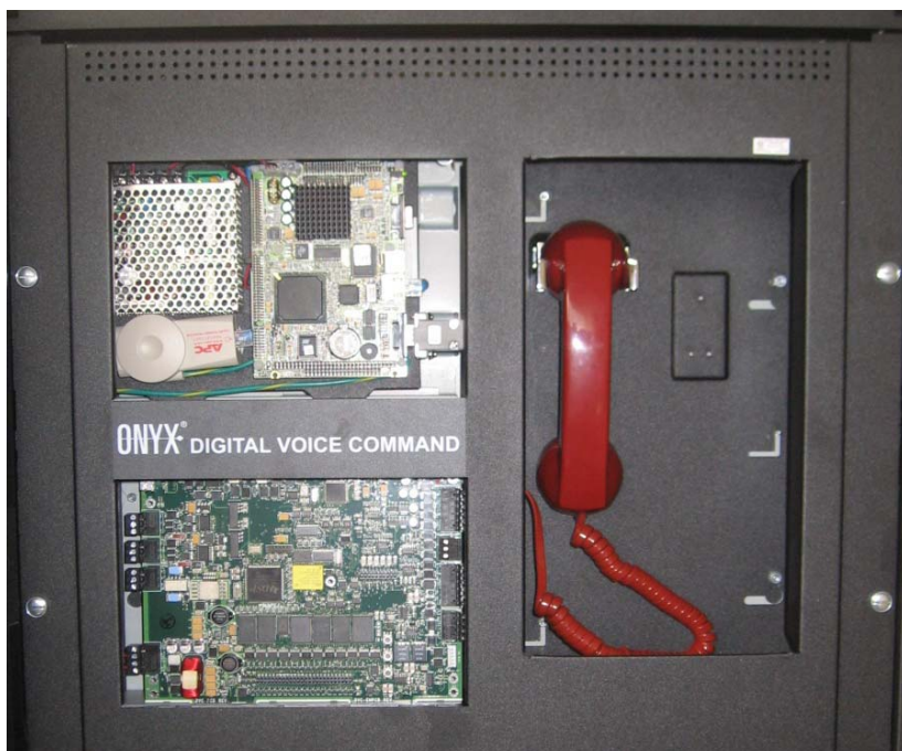
Figura 5.4. – Cabina de Bacnet Gateway.
