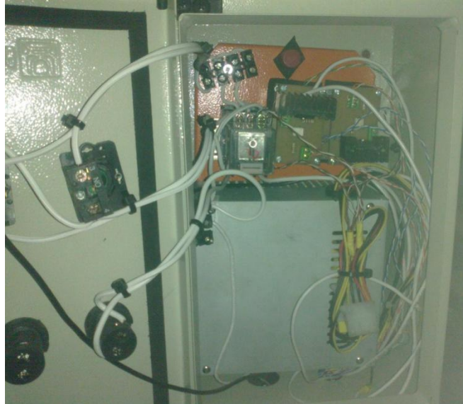
Figura 2.19: Interior del panel de control
